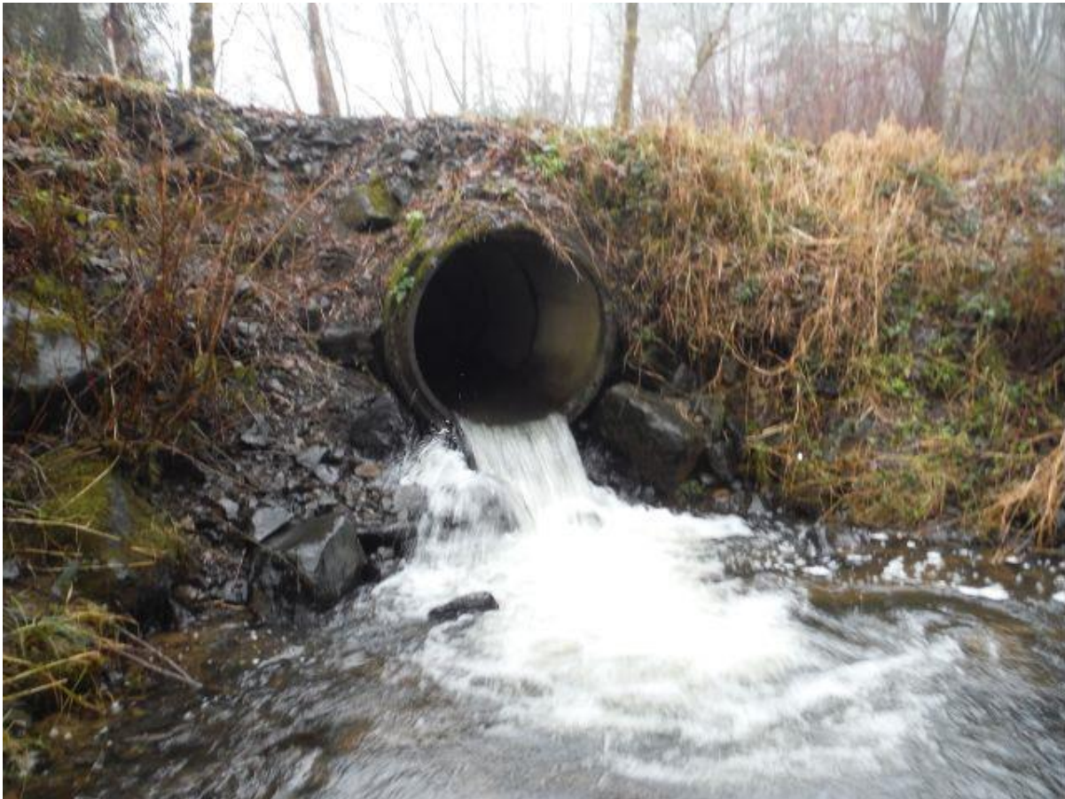
Photo: Fish passage barrier culvert. Credit: Washington Department of Fish and Wildlife.
