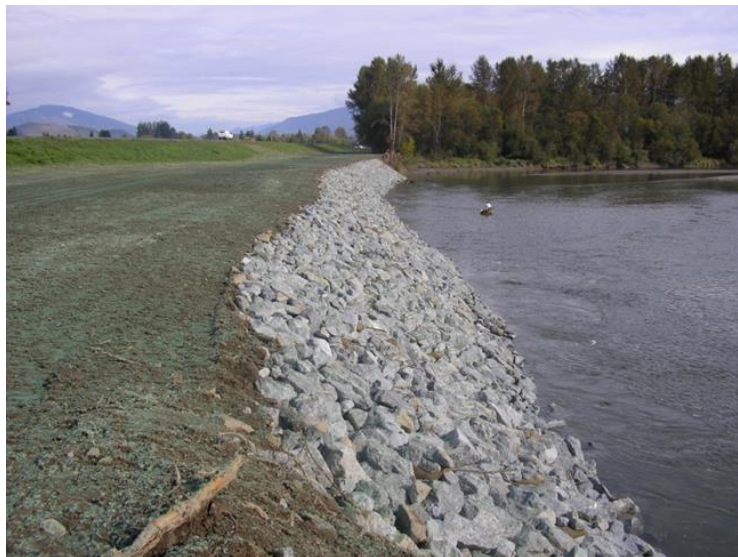
Photo: Skagit River levee isolating the river from the floodplain. Credit: NMFS.
