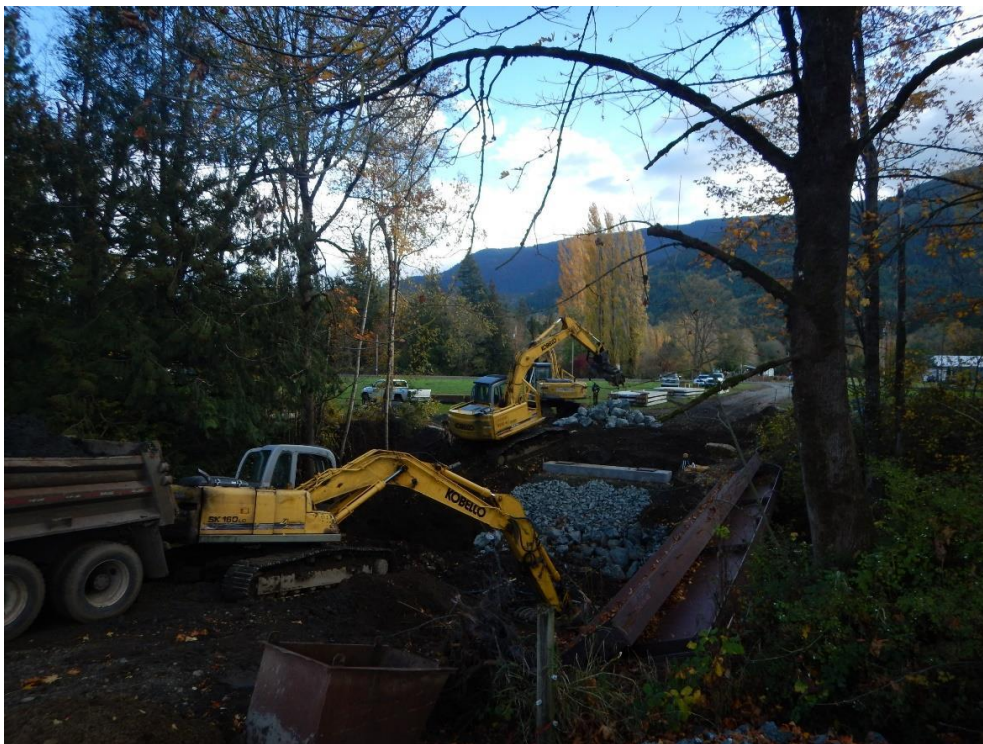
Photo: Culvert replacement for fish passage restoration. Credit: Nooksack Salmon Enhancement Association.
