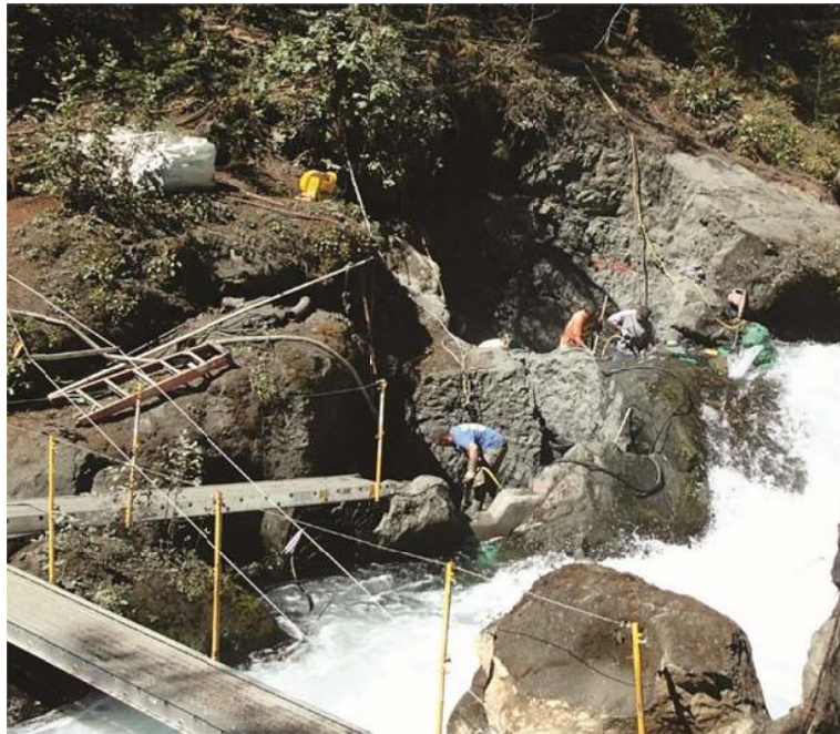
Figure 4-11. Workers completing modifications to Little Falls to improve passage for upstream migrants.
