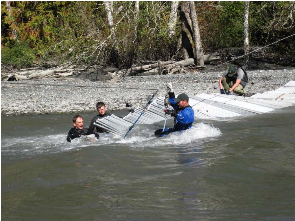
Figure 6. High river flows on August 7, 2013 made installation more challenging and operations more difficult (personnel safety was a major concern).
