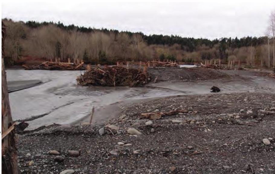
Newly constructed engineered logjams in the lower Elwha River. The structures are designed to split flows, activate new side channels, create pools and sort gravels.
