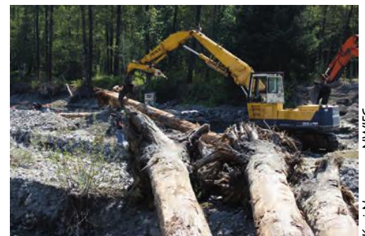
A crew installs an engineered logjam on a former tree farm acquired by the Stillaguamish Tribe.
